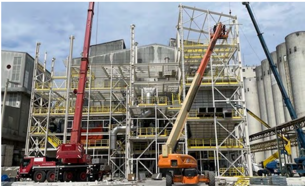
Slika 2. Dogradnja pogona SPC, nova linija za proizvodnju SPC Figure 2. Plant upgrade SPC, new production line SPC
